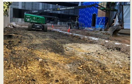
Storm water infrastructure
