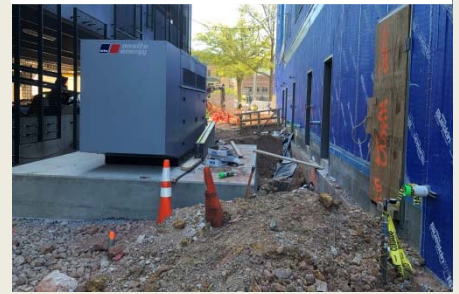
Standby Generator installed
