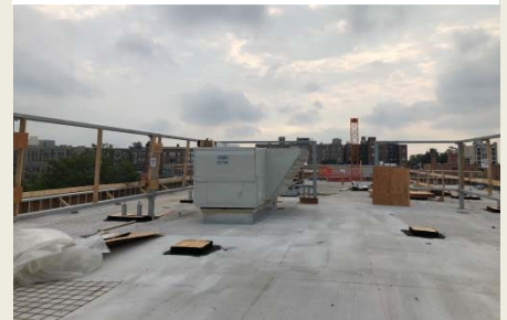
Mechanical roof top unit
